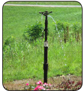
Figure 45. Ensure nozzles are working properly
