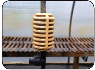
Figure 16. Iron deposits can easily clog an irrigation or a mist system
