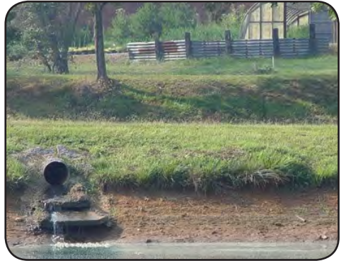
Figure 1. Irrigation pond below desirable water level
