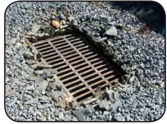
Figure 55. Drainage tiles lead to underground pipes that carry water to the containment structure
