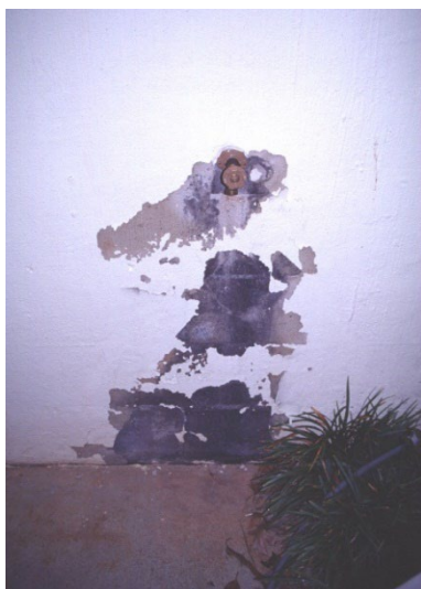
Figure 5. Repair plumbing leaks as quickly as possible. Moisture attracts termites to the structure.
