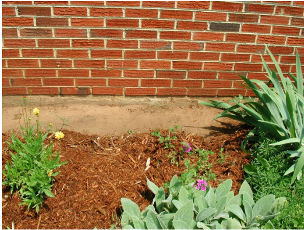
Figure 4. Leave a 12- to 18-inch bare zone (i.e., pull back the mulch next to the foundation to prevent providing a bridge to subterranean termites over the termiticide-treated zone).
