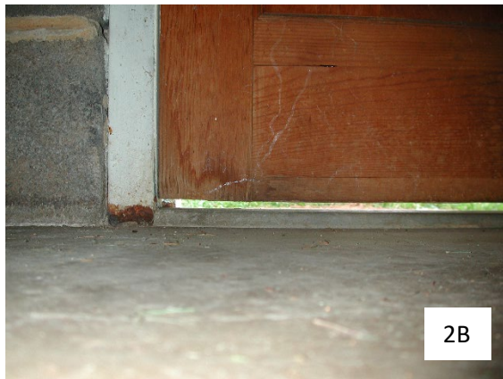
Figures 2a and 2b. Gaps around doors should be sealed.
