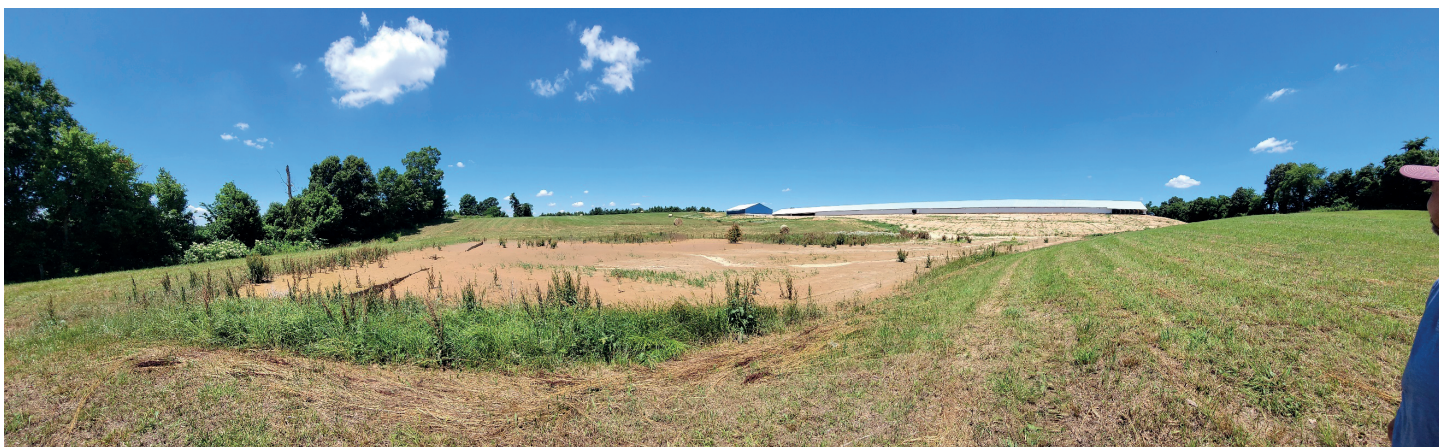
Figure 6. Panoramic photograph of an 8-house broiler farm where the barn construction was recently completed. The engineered sediment basin in the foreground (silt fence partially visible) is filled to overflowing with sediment. Sediment was discharged offsite and was in part deposited onto a neighbor's field. The sediment was composed of soil washed from a construction site with highly erodible soils. The grading contractor did not implement erosion prevention and sediment control practices, including the critically-needed permanent vegetation.
