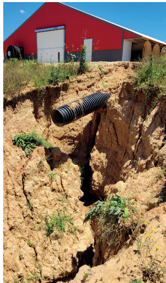
Figure 5. Massive gully erosion at a drainpipe without outlet protection.
