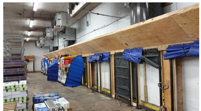
Figure 16. Cold wall with several single pallet cooling bays. Photo: S.A. Sargent
