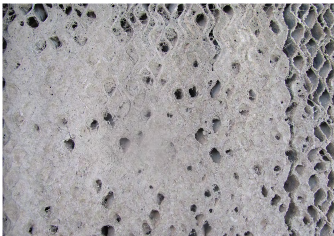
Figure 4. Mineral buildup has clogged much of this cool cell pad. Source: Tom Tabler
