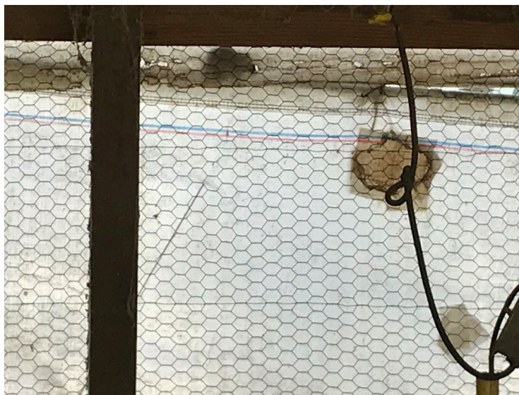
Figure 3: Rodent on top of roof
