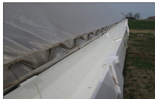
Figure 3: Plastic snap together gutters on a high tunnel. Repair tape was used to fill the gap between the gutter and the structure.
