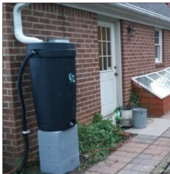
Figure 1: Small-scale rainwater harvesting is becoming more common in residential areas.
